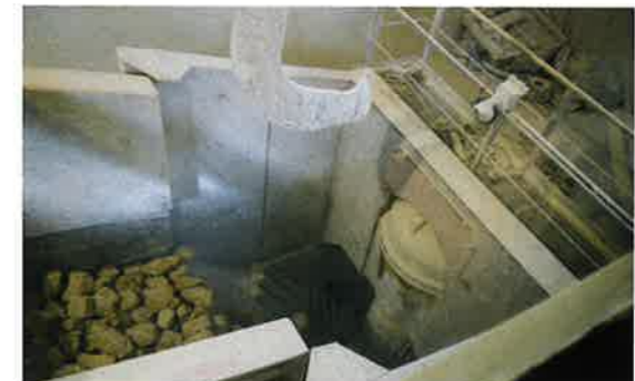
Fig. 7: Jaw crusher to be connected to the Bielomatik automatic grease supply
