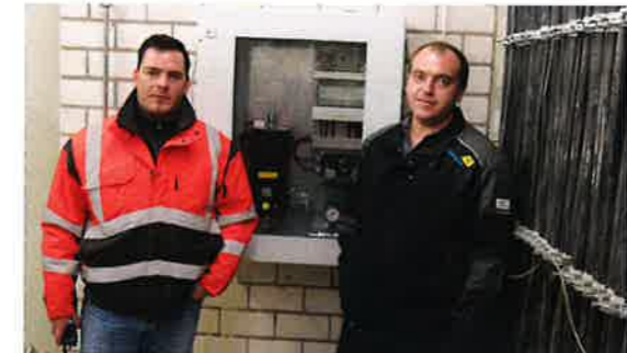
Fig. 6: Operations manager Toni Pranghofer and service technician Oliver Oswald in front of a dust-proof electronics cabinet with glass control window
